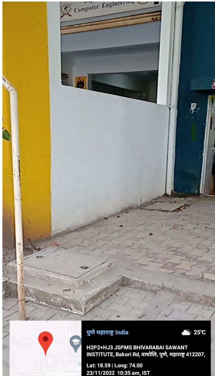
Fig. 5 Rain water storage
