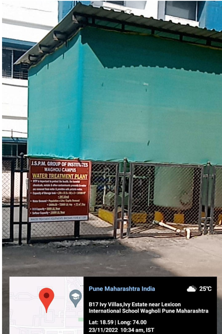
Fig. Water Treatment Plant at at ICOER
