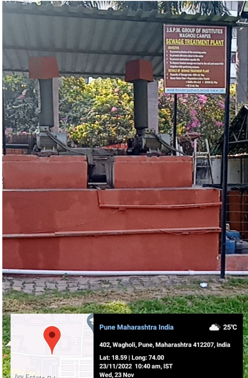
Fig. 6 Sewage Treatment Plant at ICOER
