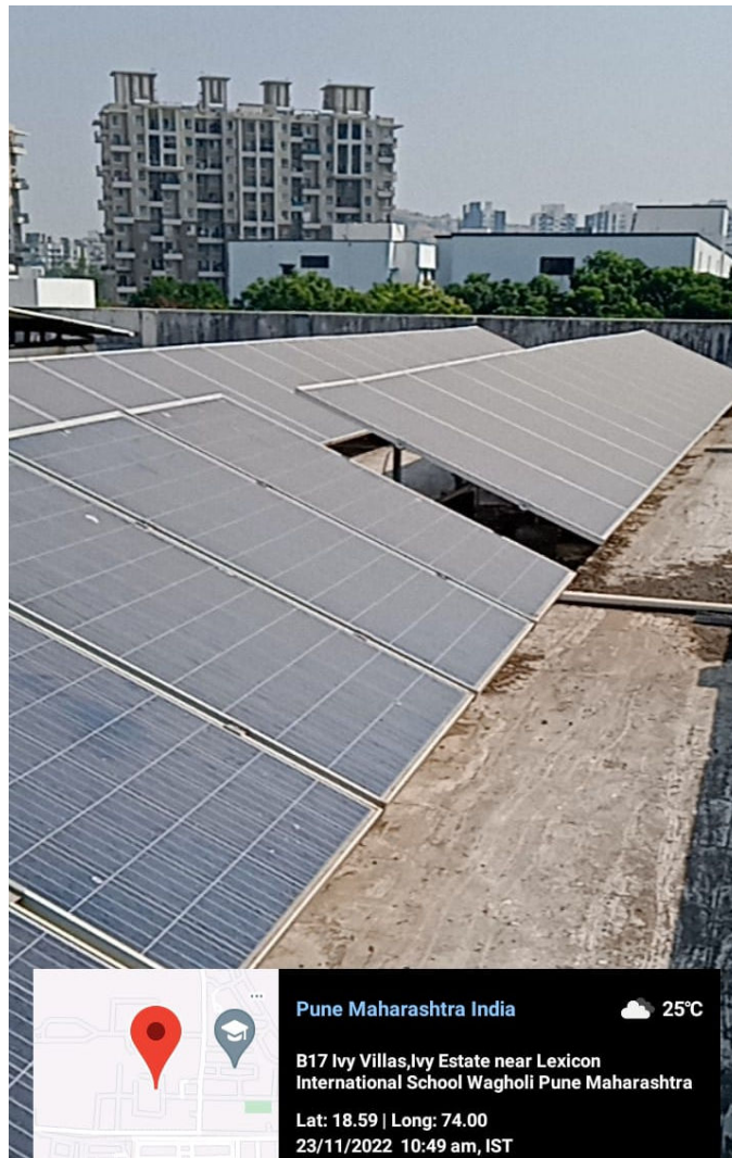
Fig. 1 Solar panle on roof of building-C
